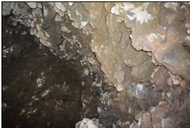
Fig. 7. Void 2 - shattered rock ceiling.
