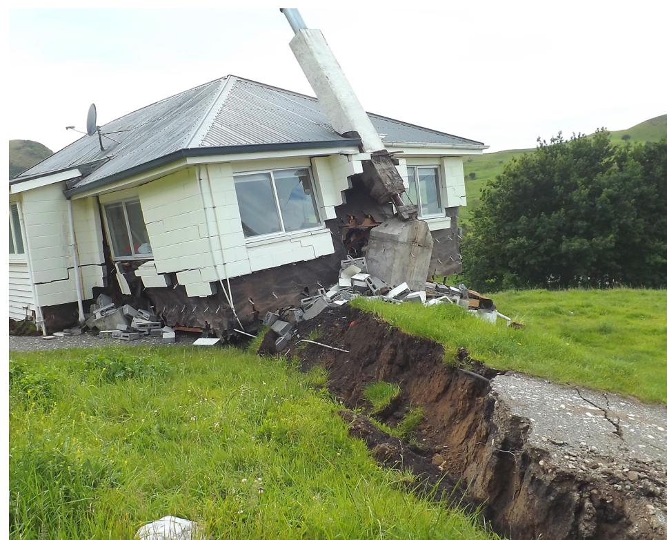
A damaged house along the Kekerengu Fault.
